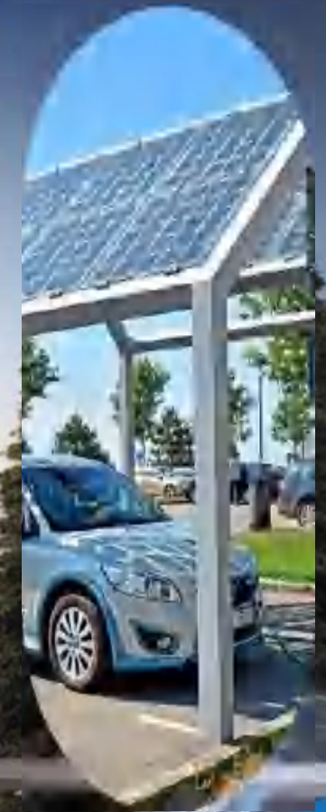
EV Charging Station
